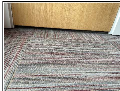
Issue ID Reference: 4.1 Example threshold gap to compartment fire door.
