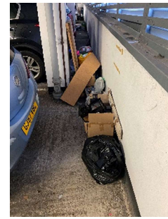
Issue ID Reference: 2.3 Example of combustibles in the car parks.
