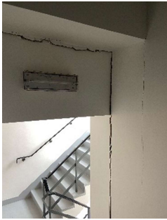
Issue ID Reference: 4.4 Example of compartment wall cracks along stairwells.
