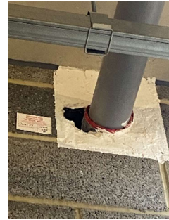
Issue ID Reference: 4.5 Damage to fire stopping in plant room.
