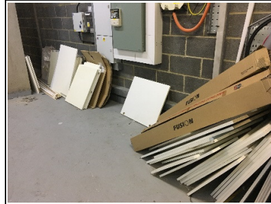
Issue ID Reference: 2.1 Combustibles in the plant room.
